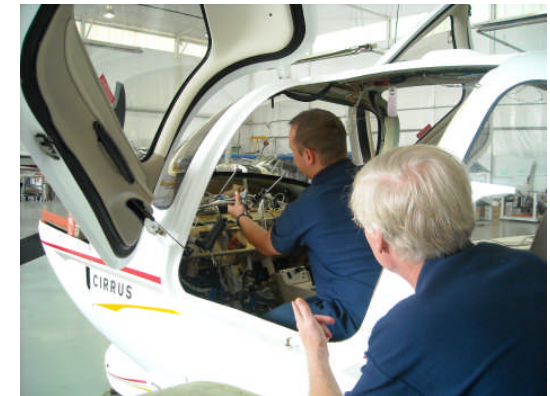
Dustin Moeller and Jack Musgrave beginning the installation of Avidynes's Release 9 Integrated Flight Deck in Gil Williamson's Cirrus SR22 N426GW.
